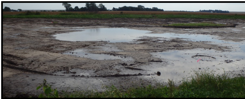
The picture above is the start of the wetland excavation to create the shallow water wetland.. Next the area will be seeded.
